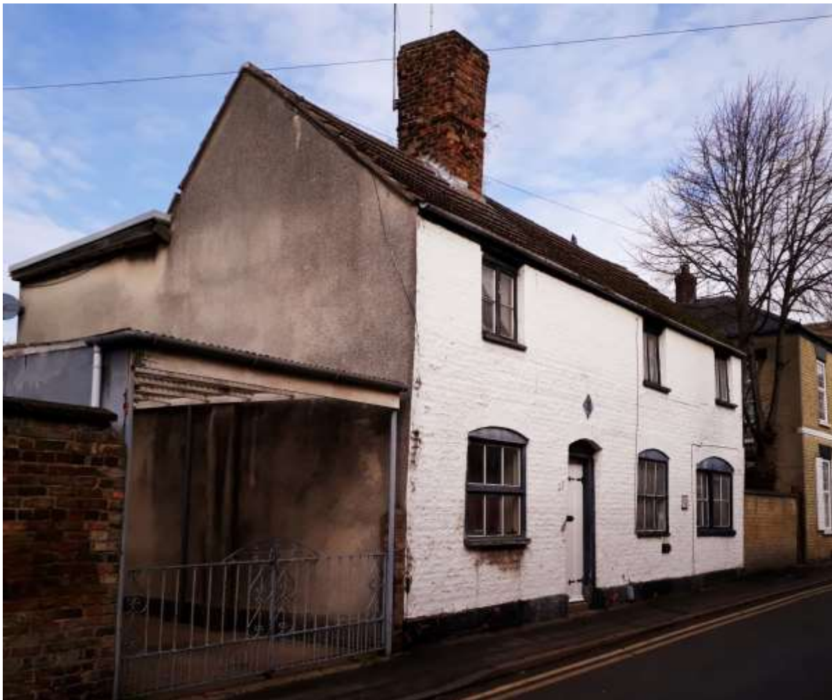
20-22 St Mary's Street is probably the oldest surviving building on the street but its front elevation and stack are in need of repair and maintenance.
