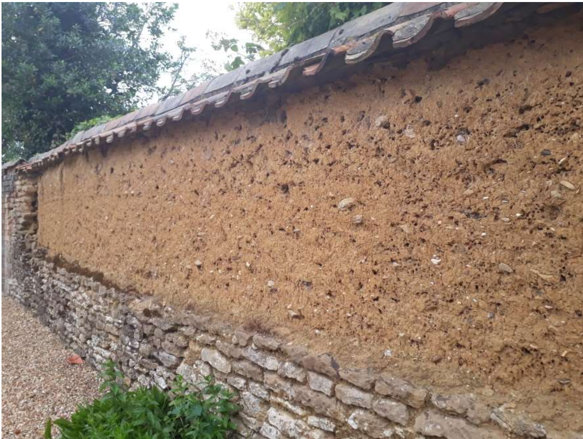
The Mud Wall between 8 Delph Street and Delph Court is an example of a fine mud wall serving as a side boundary and hidden from view from the street.
